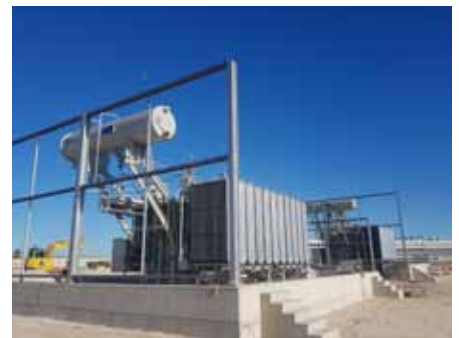
Australia, 3 PHASE 132kV 45MVA
