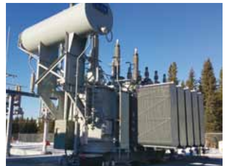
CANADA, 3 PHASE 138KV 42MVA
