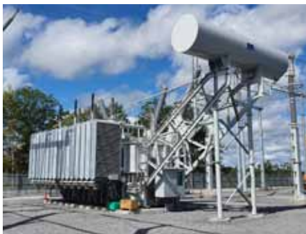
USA, 3 PHASE 500KV 350MVA
