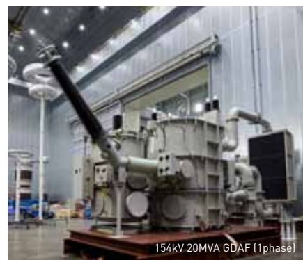
154kV 20MVA GDAF [1phase]
