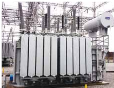
USA, 3 PHASE 345KV 448MVA
