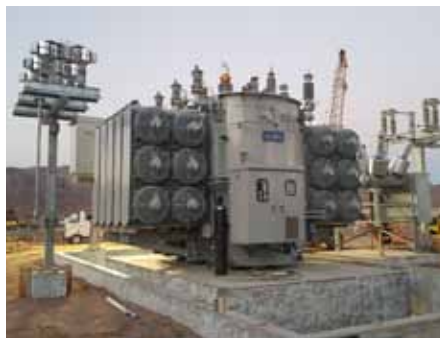
USA, 3 PHASE 69kV 150MVA
